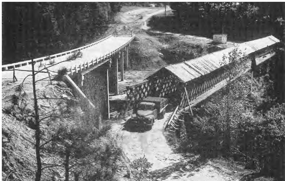
In 1955, the Association’s magazine printed this photo of a Farm-to-Market program project, with a modern concrete bridge taking shape alongside the covered wooden structure it was replacing.
